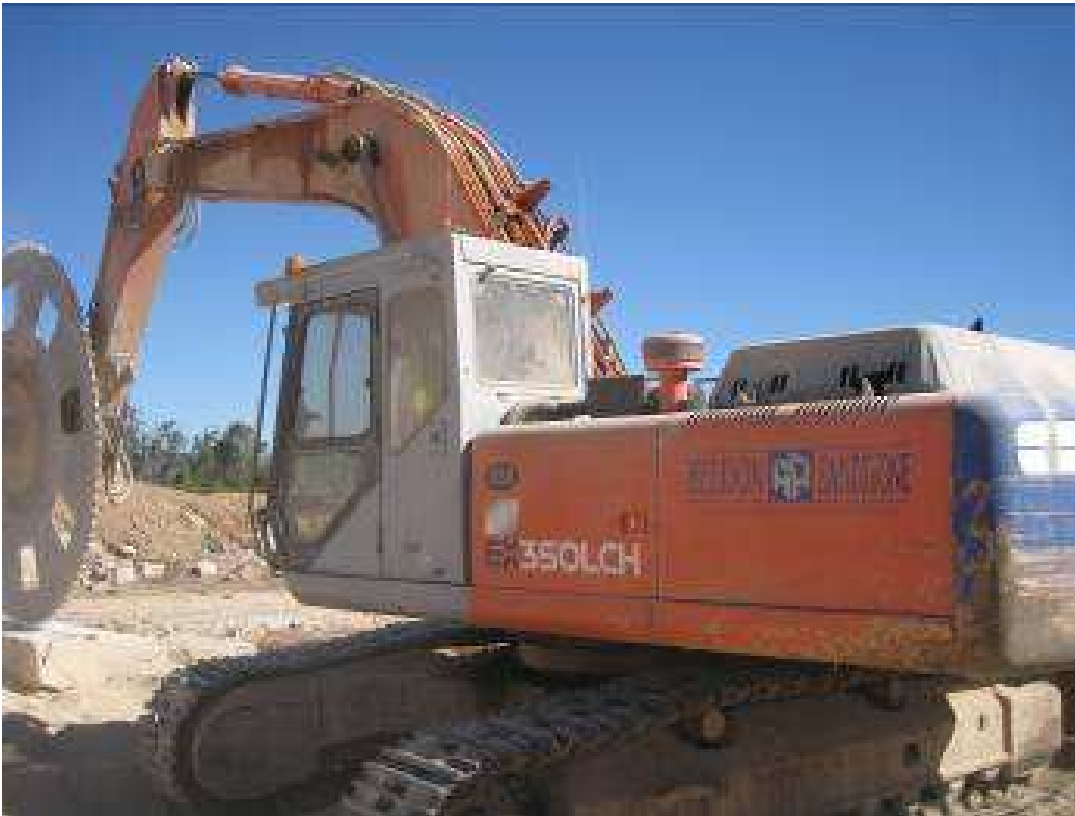
Photograph # 2; 350 LCH excavator, with saw attachment, cutting sandstone with RESPA™ SD unit installed (mounted behind cabin).
